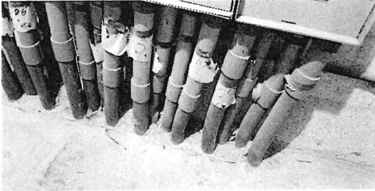
Emergency Lighting/Exit Lights.
