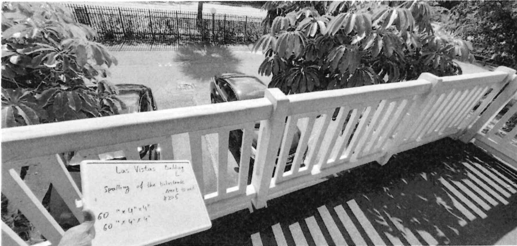
Photo 7 : Spalling of the balustrade next to unit #205.(60"x4"x4").
