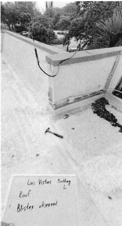
Photo 10: Roof - Blister Observed
