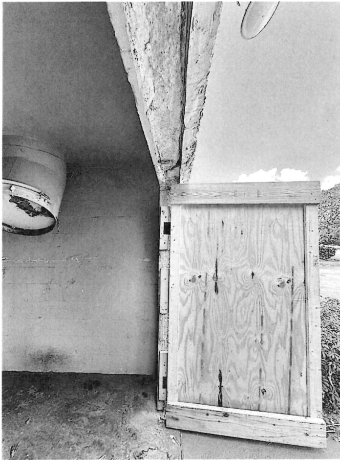
Photo 30: Make shift Polywood & 2x6 wood framed Garbage/Trash room door; (replace) with approved metal 2-Hr fire door as per code.
