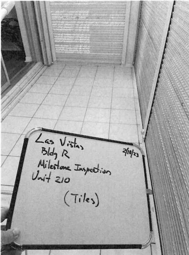
Photo12 : Tiles at unit 210 balcony.
