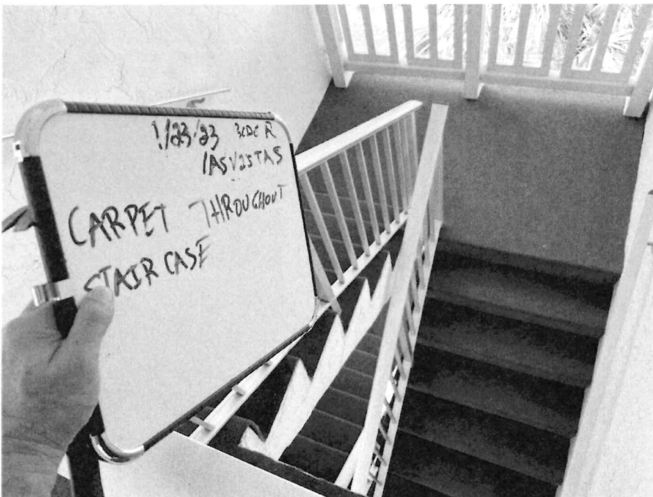
Photo 5: carpet Staircase throughout, recommended removal of carpet.
