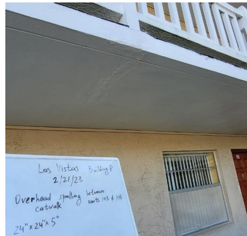
Overhead spalling between Units 103 and 104
