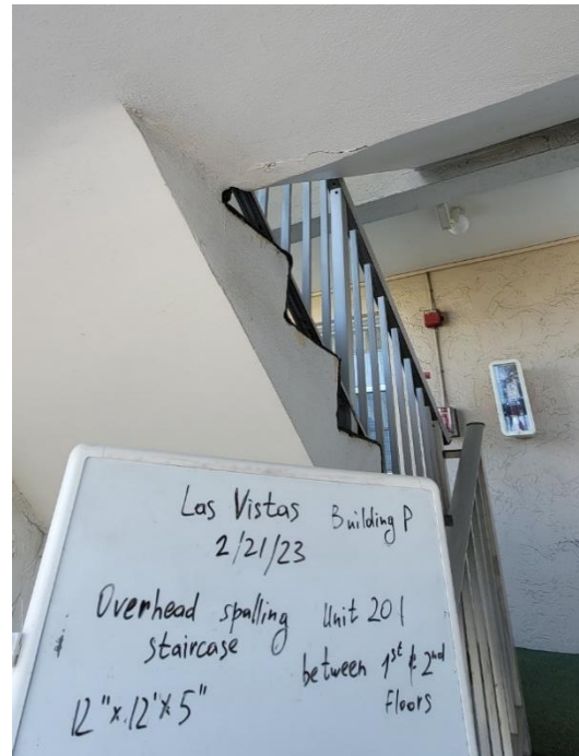
Overhead spalling on staircase between 1 st and 2 nd floor (Unit 201)
