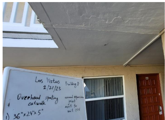
Overhead spalling around expansion joint next to Unit 205
