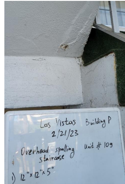
Overhead spalling on staircase in front Unit 109
