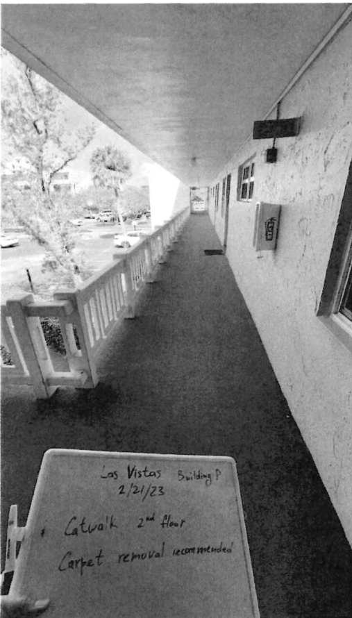
Photo 6: Catwalk second floor- Carpet removal recommended.
