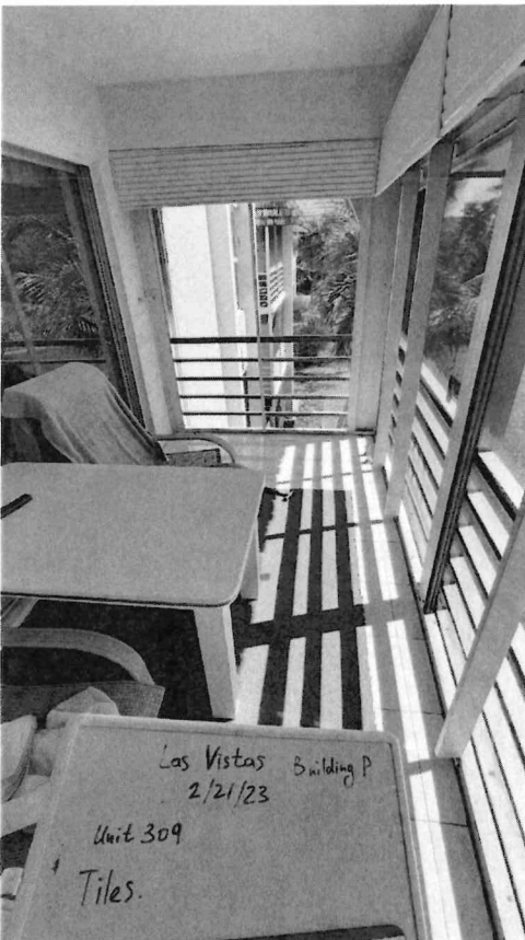
Photo 8: Tiles at unit 309.
