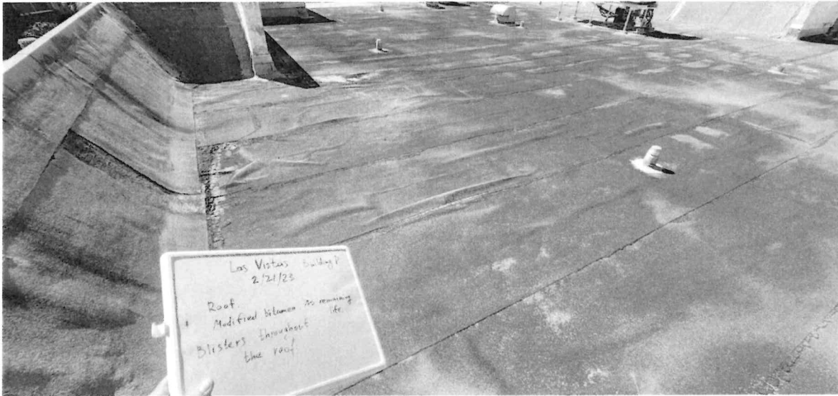
Photo 12: Roof Modified Bitumen no remaining life - Blisters throughout the roof. Roof replacement recommended.
