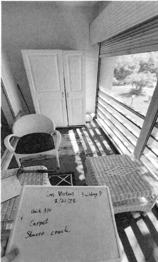
Photo 7: Carpet - stucco crack, unit 310.
