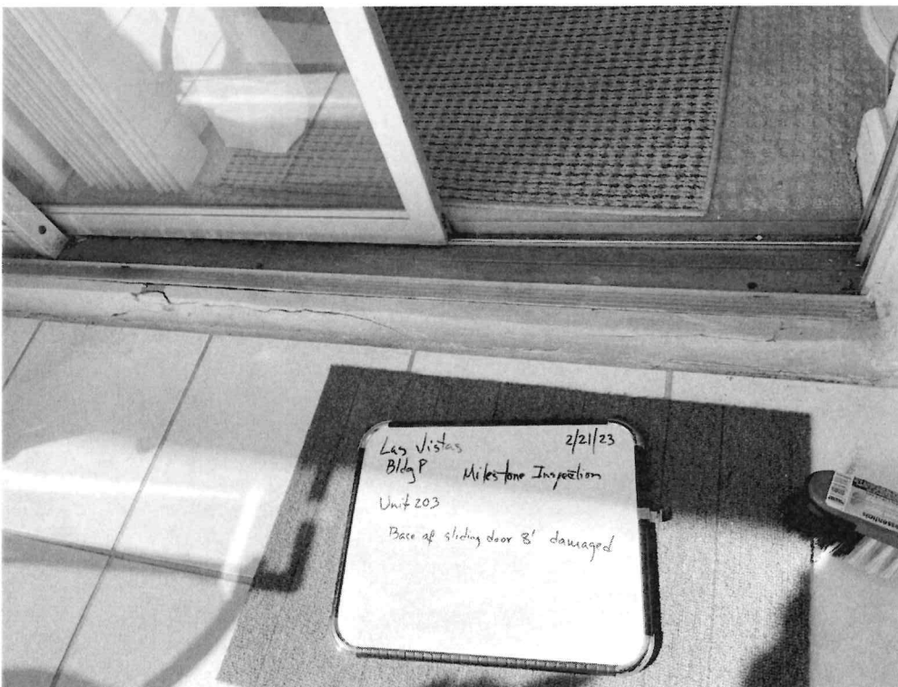
Photo 17: Unit 203 base of sliding door 8' cracks/spalling damage
