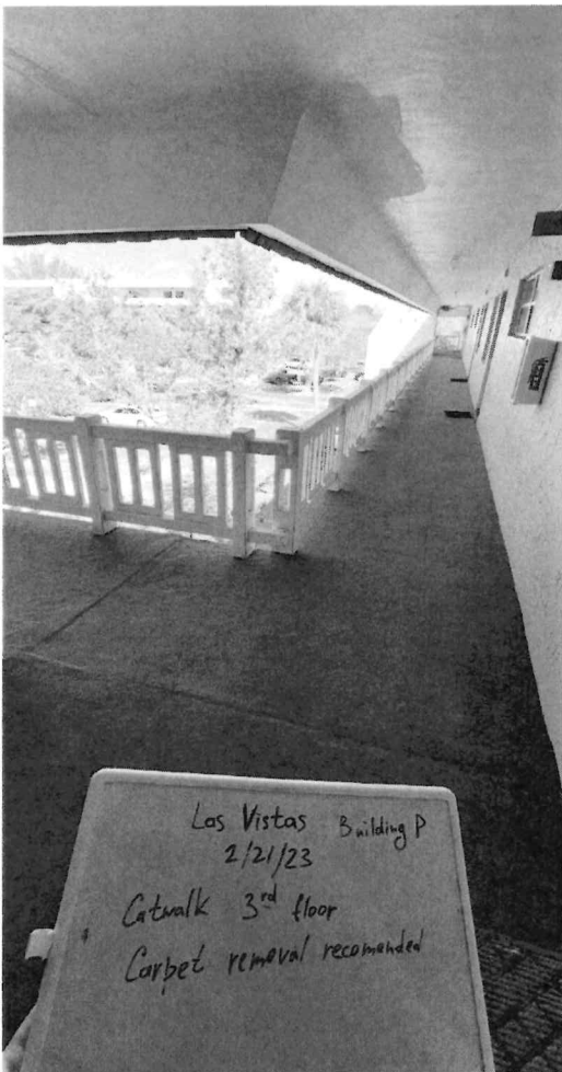
Photo 13: Catwalk carpet removal 3rd floor recommended.
