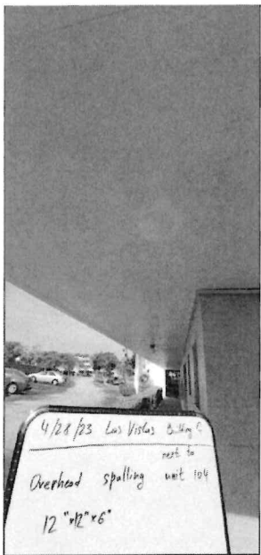
Photo 8: Concrete catwalk overhead spalling next to unit #104.
