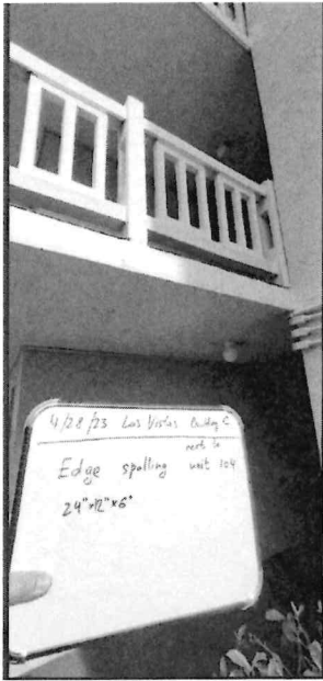
Photo 8 : Concrete catwalk edge spalling next to unit #104.
