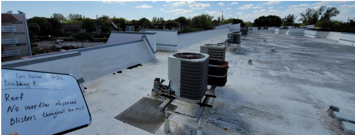
Roof: Blisters were observed throughout the roof. It must be replaced.
