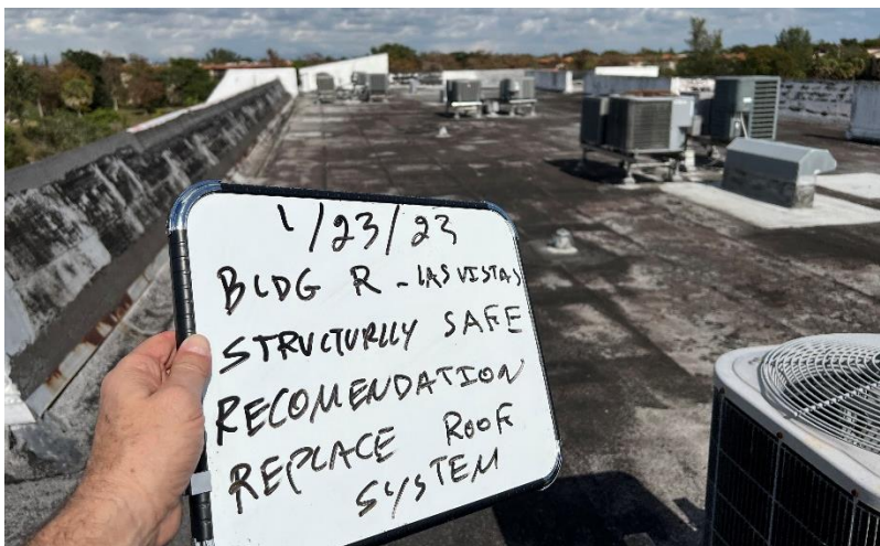
Roof with no remaining life (parapet walls and roof in poor conditions)
