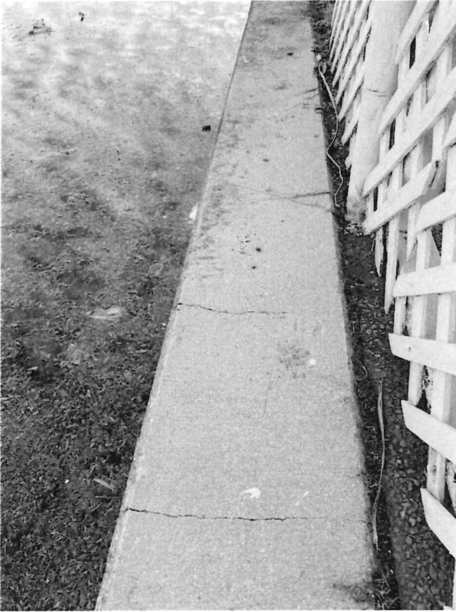
Photo 17 : Sea wall: observed several cracks at top of concrete cap north side. Repairs required to seal cracks.
