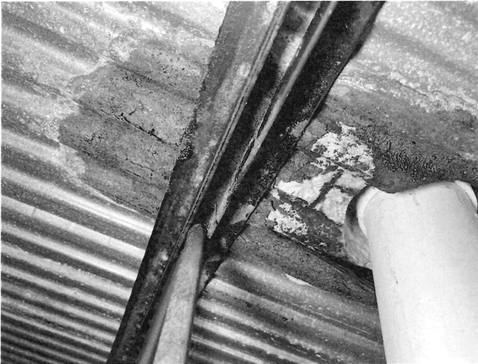
Photos: 11&12: Rusty flat roof corrugated metal deck that must be repaired or replaced. Also observed rusty open web steel joist top section.
