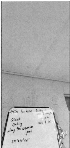
Photo 8: Concrete catwalk spalling near expansion joint next to unit #107.
