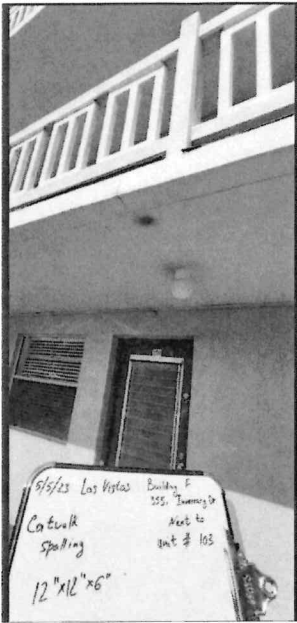
Photo 8 : Concrete catwalk spalling next to unit #103
