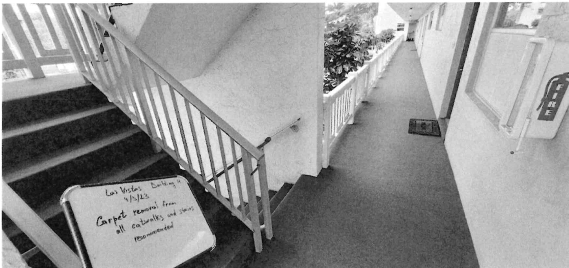
Photo 12: Carpet - Removal from all catwalks and stairs recommended
