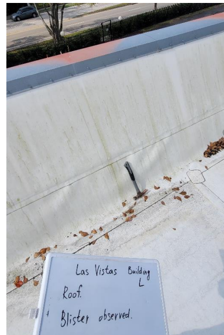
Roof (Single-ply roofing system with blisters)
