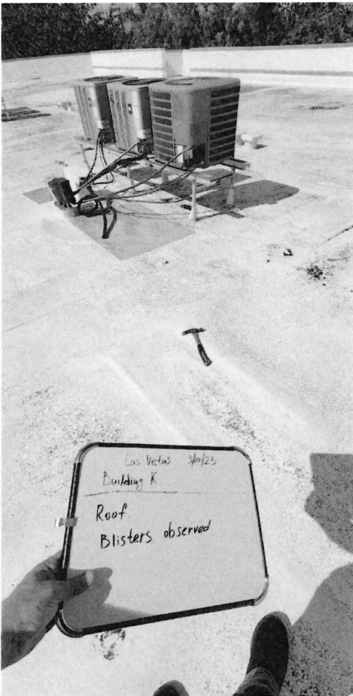
Photo 18: Roof Blisters observed.
