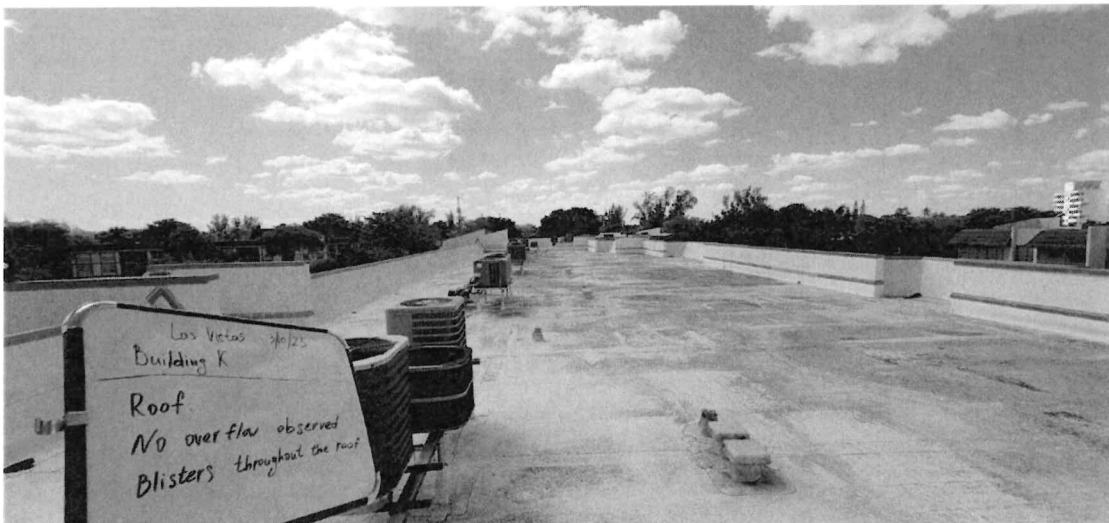
Photo 20: Roof No overflow observed & Blisters evident throughout the roof.
