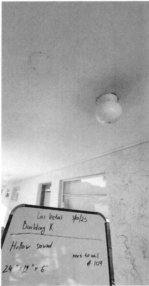
Photo 7: Hollow sound ceiling plaster/stucco: 24"x12"x6" next to unit 109
