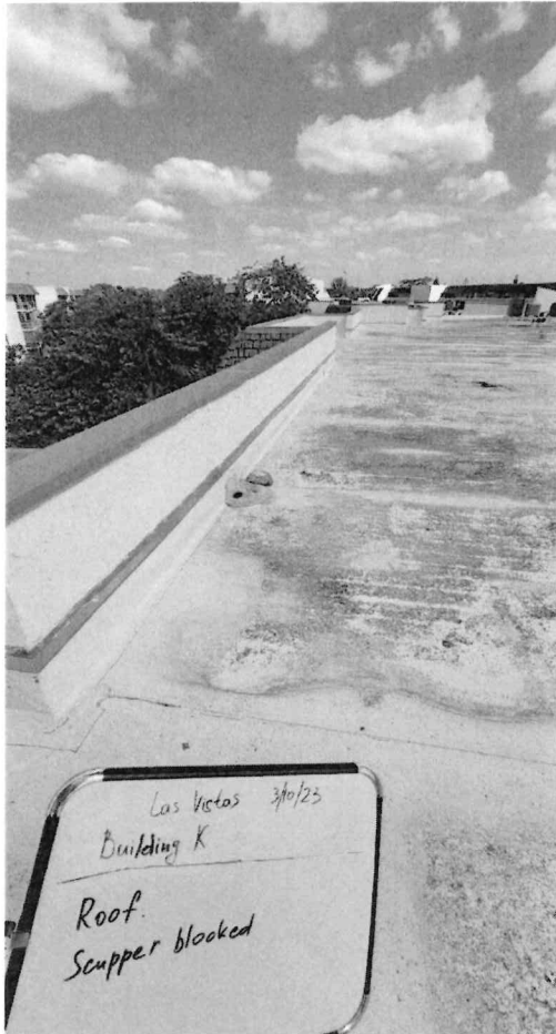
Photo 19: Roof Scupper Blocked
