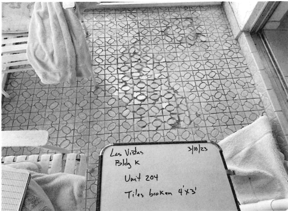
Photo 23: Tiles broken observed at unit 204, 4'x3'
