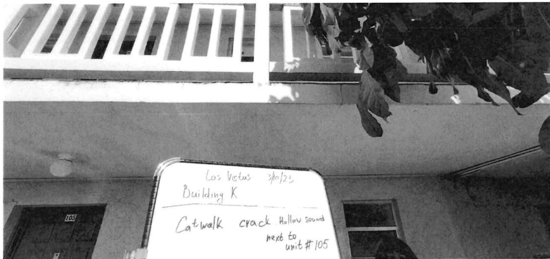
Photo 12: Catwalk slab edge crack. Hollow sound next to unit 105.
