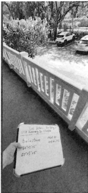
Photo 7 : Concrete Rail cracks ( Balustrade) next to unit #206.
