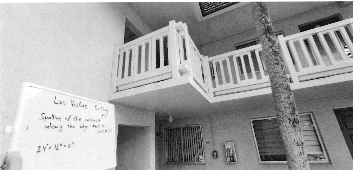
Photo 7: Spalling of the concrete catwalk along the edge next to unit #101; 24"x12"x6"
