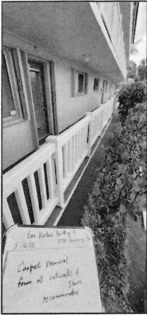
Photo 7: Concrete catwalk edge spalling observed. Carpet removal from all Catwalks and stairs recommended.
