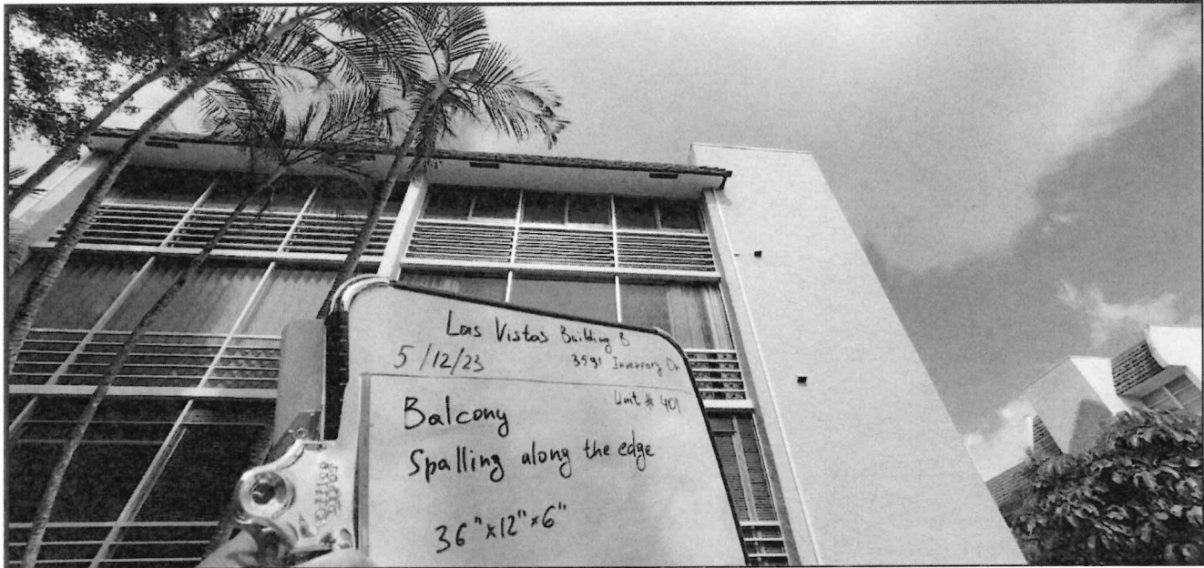
Photo 9 : Concrete balcony edge spalling next to unit #401.
