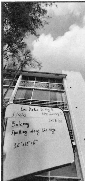
Photo 10 : Concrete edge of balcony spalling next to unit #401.
