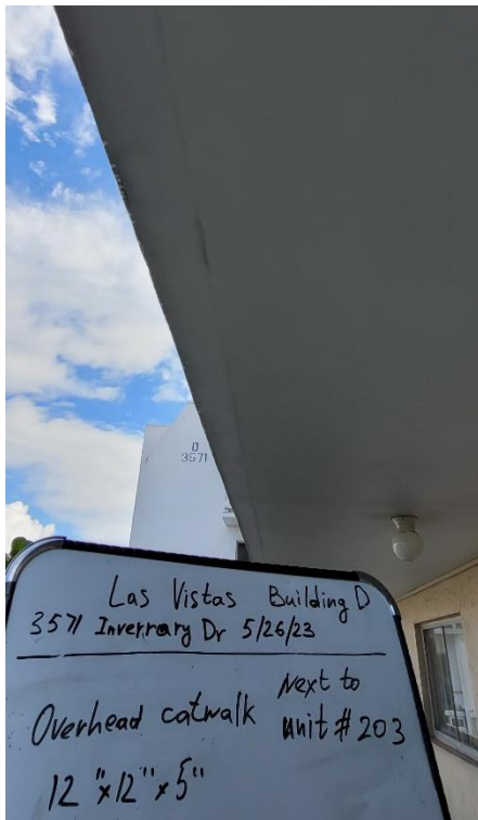
Next to Unit 203
