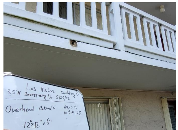
Next to Unit 108
