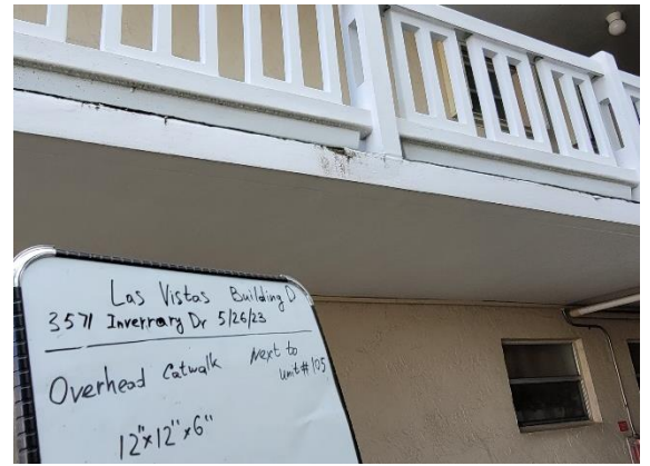
Next to Unit 105
