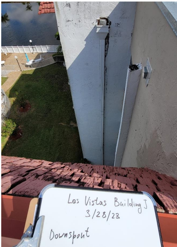
Roof: Downspout broken
